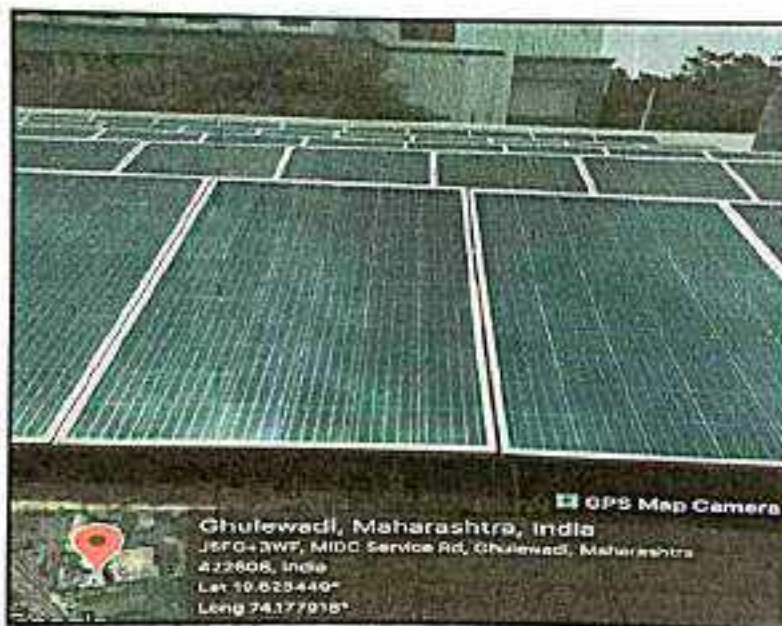
Photograph of Roof Top Solar PV Plant:
