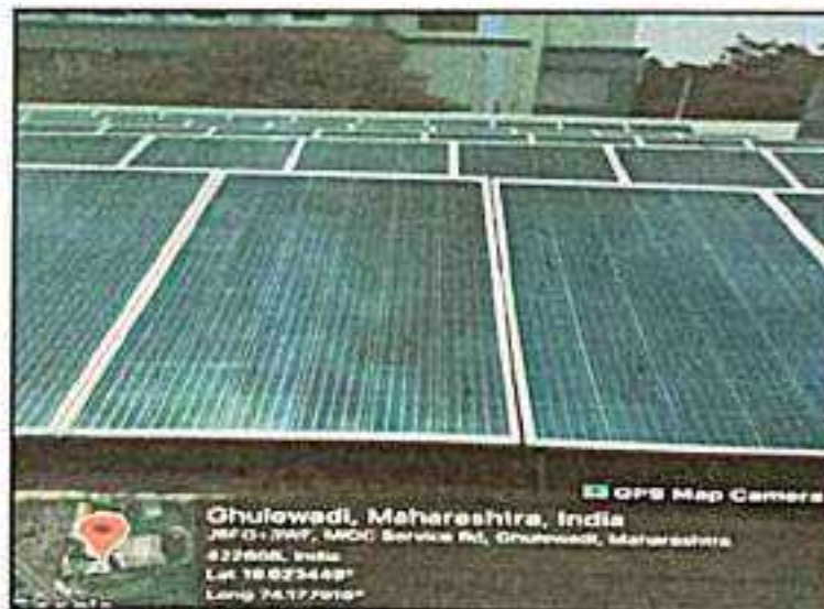
Photograph of Roof Top Solar PV Plant:
